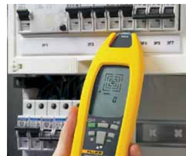
Location of fuses/breakers and assignment to circuits
