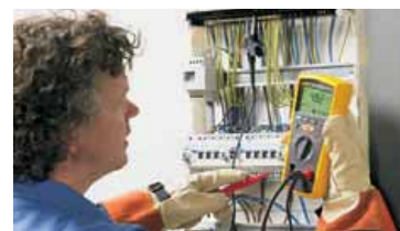
Insulation test at a distribution panel
